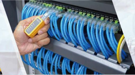
◆ Copper Cabling system
